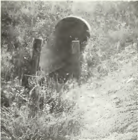
EAST ENTRANCE - Water in pipe
